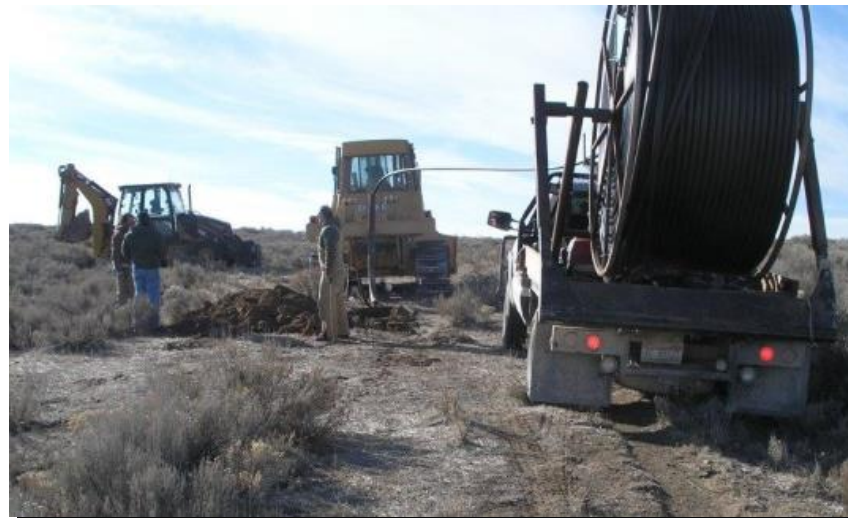
Three deep wells and 42 miles of pipeline
